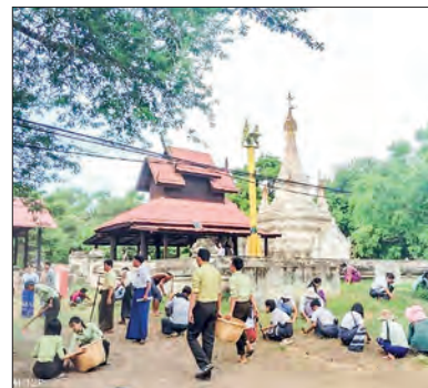
Workers clear vegetation within 20 feet of ancient monuments at the Bagan World Heritage Site.
